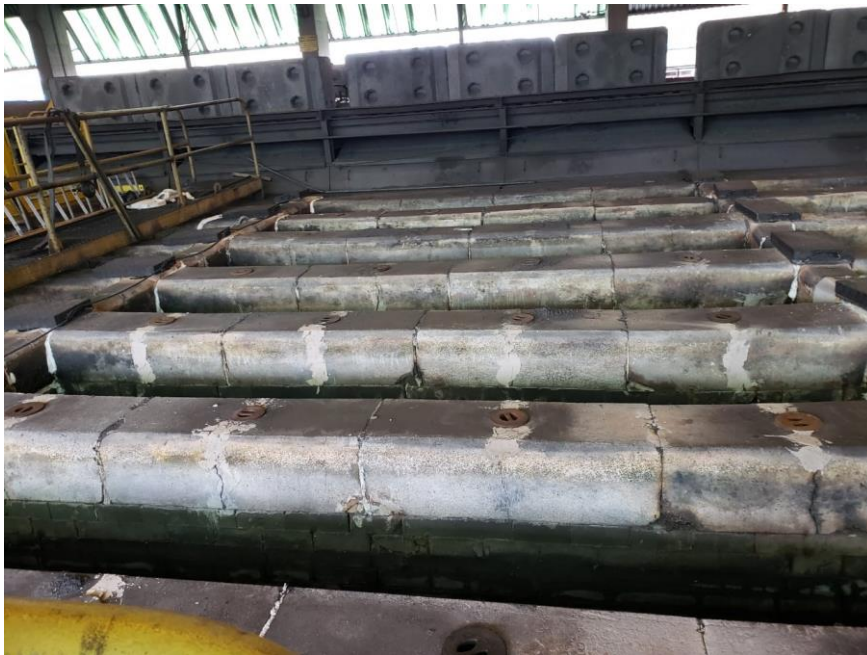
Figure 4 - Cracks observed in top blocks after years of continuous operations.
